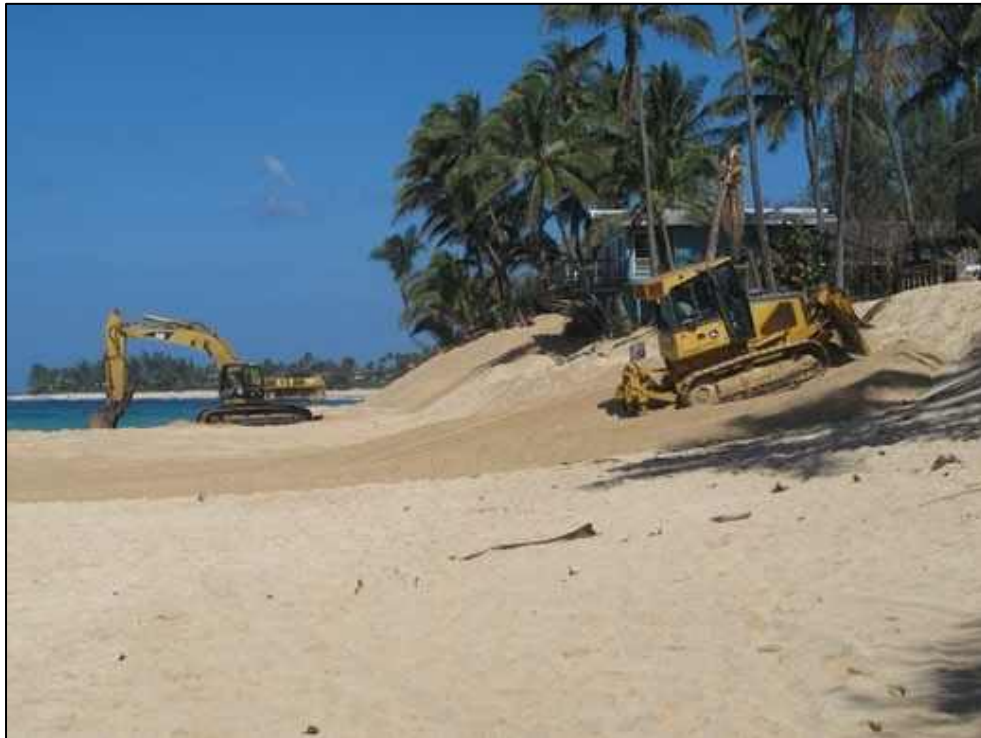
Figure 3-1 Sand pushing at Sunset Beach, O‘ahu (2014)
